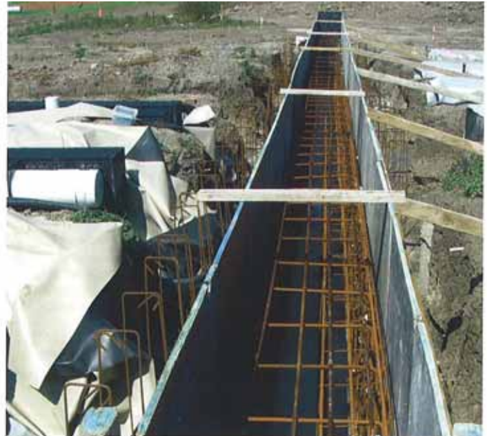
Above: Most of the ventilation ducts will be connected to large inlet funnels, but one classroom requires a ventilation plenum, seen here under construction.
