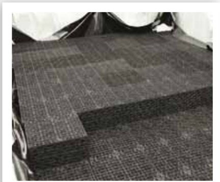
CelluTank® Re-use System Hawthorn Victoria.
