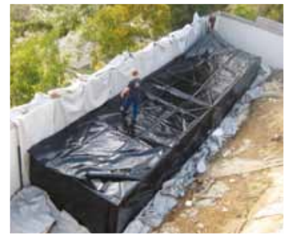
CelluTank® Re-use System Eaglemont Victoria.
